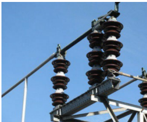
115 kV Disconnect Support
