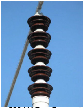
230 kV Bus Support
