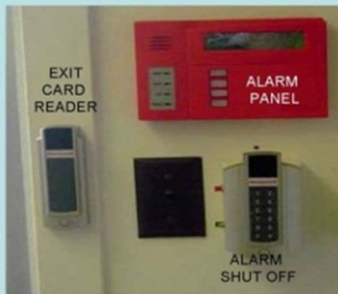
Figure 7. Recommended Labeling of the Alarm Card Readers inside the BPA Facility
