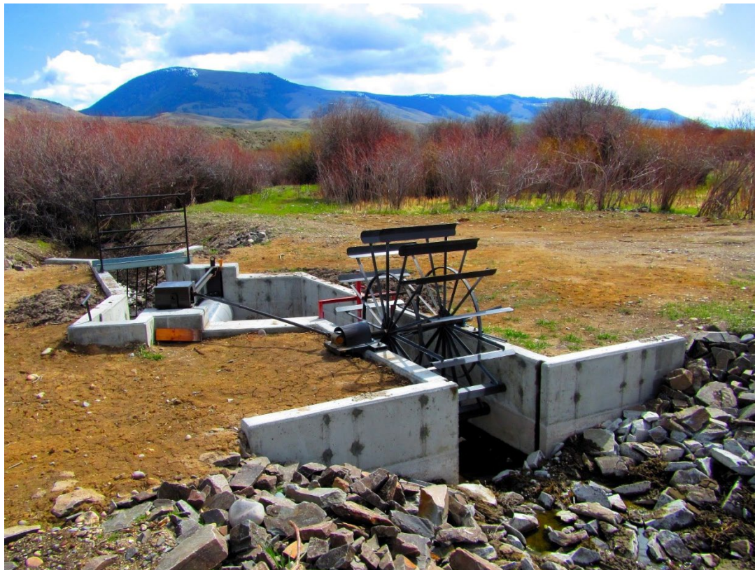
Figure 33:2023040 Upper Salmon Fish Screens
