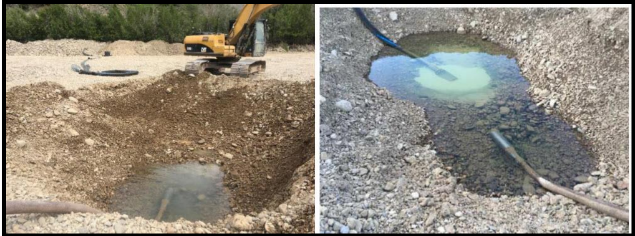
2019012 (Yankee Fork) pumps used to lower groundwater table to prevent turbid water from percolating through the mine tailings to Yankee Fork.
