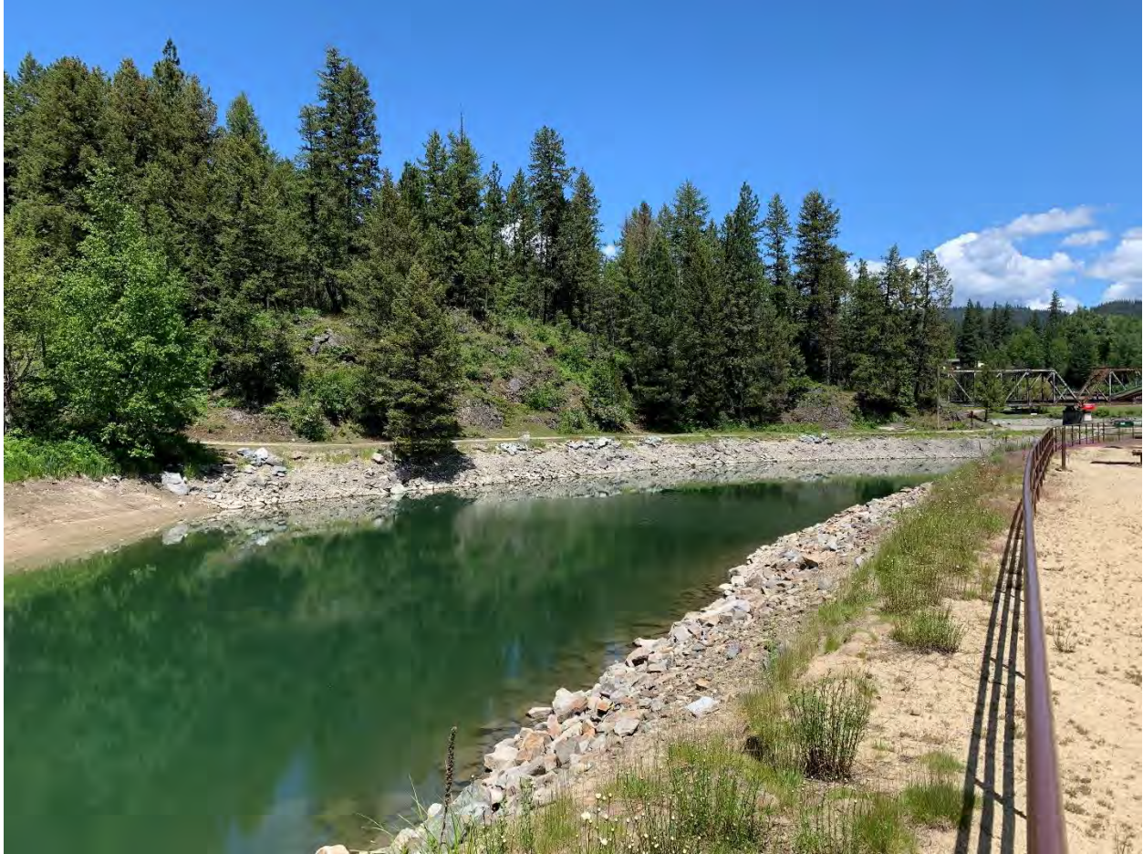
Figure H-6. Image of the Albeni Cove riprap. This area was identified as a place that needed bank stabilization repairs for FY 2022. The photograph is a “before” picture (spring 2022).
