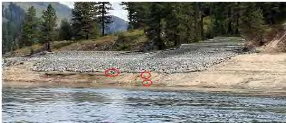
Figure J-3. Site protection/stabilization at site 45ST437 on the Mainstem of Lake Roosevelt, Washington. Note the large rocks circled in red that migrated downslope.
