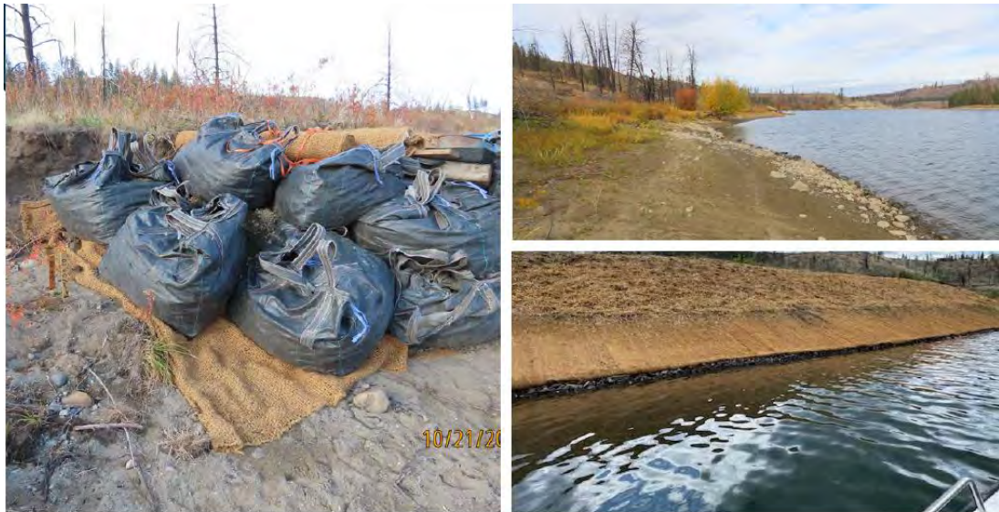
Figure J-5. Various stages of construction at site 45LI377: Phase I in FY 2021 (left); Phase 2 in FY 2022 (center); and Phase 3 in FY 2023 (right).
