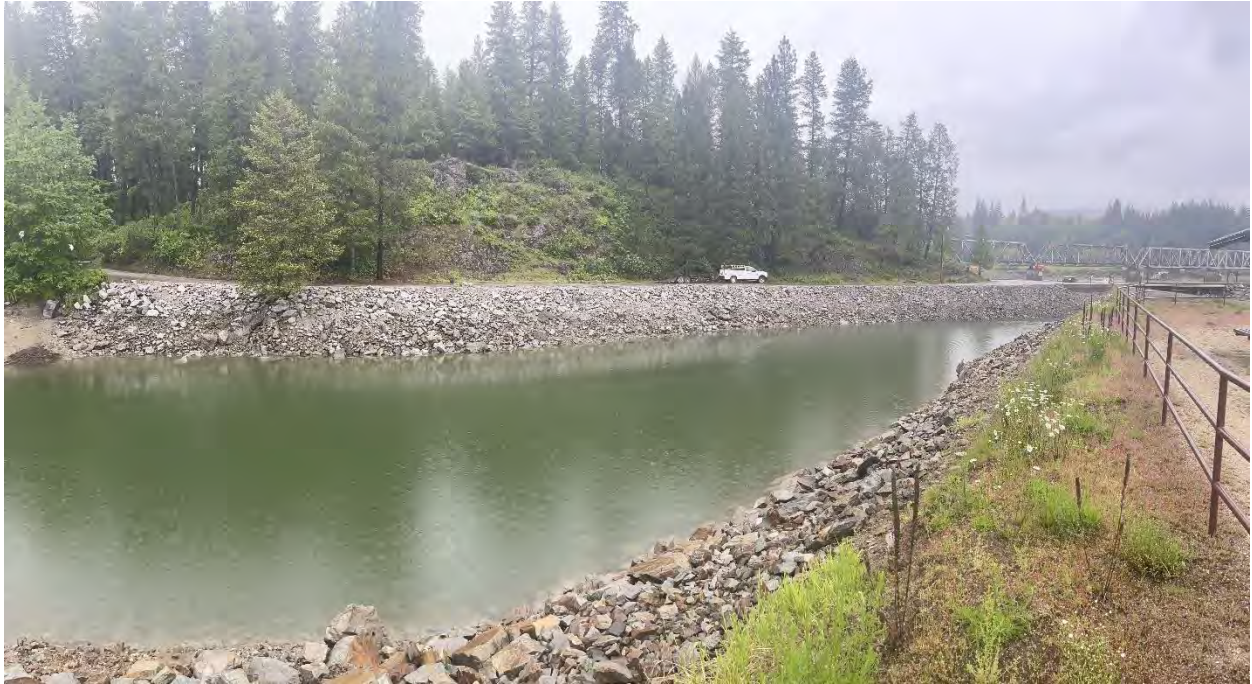
Figure H-7. Image of the Albeni Cove riprap showing the bank stabilization repairs that occurred in FY 2022 (summer 2022).
