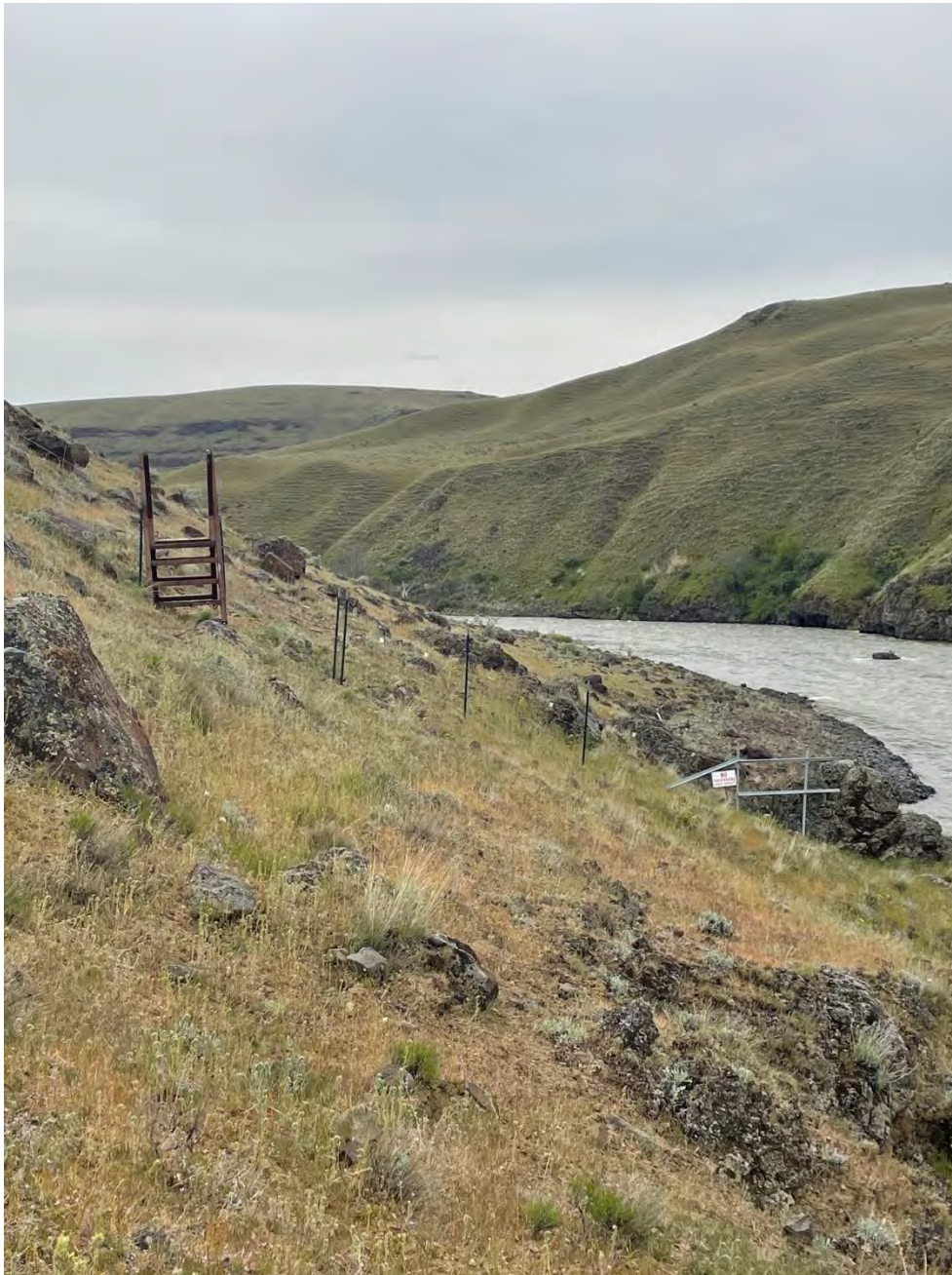
Figure E-1. New fence (completed in FY 2022) at John Day Narrows to prevent cattle from trampling eligible archaeological sites.
