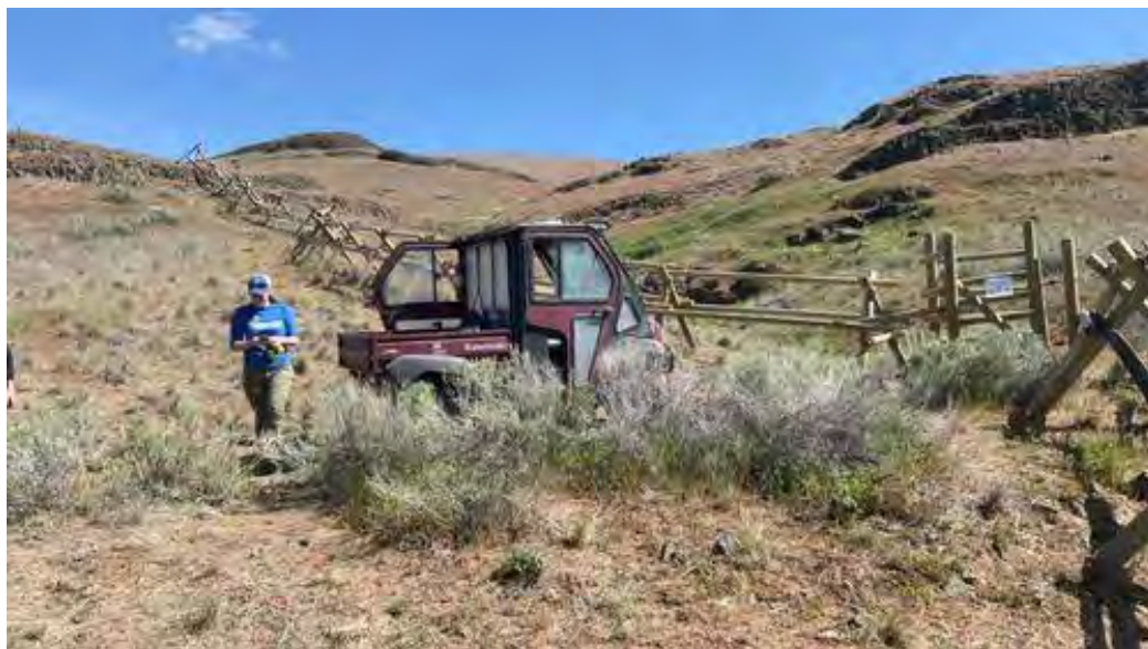
Figure F-6. Installation of a buck-and-rail fence and gate to discourage recreational impacts to a site at Lower Granite in FY 2022.
