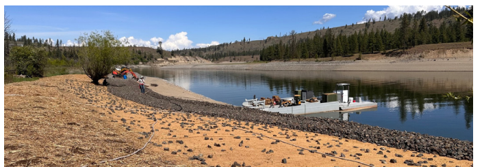
The concluding phase of a stabilization project on the Spokane River shows the expansive 900-foot-long protection system and barge used to supply materials.
