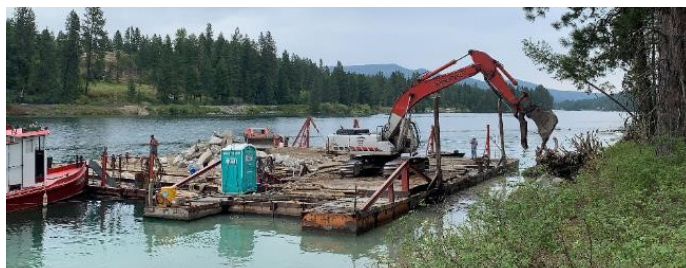
In-progress bank stabilization of a historic homestead and precontact camp site affected by erosion within the Albeni Falls Project.
