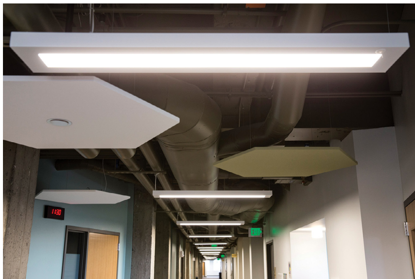
Enlighted Luminaire Level Lighting Controls installed in the Pacific Tower building in Seattle, Wash.
