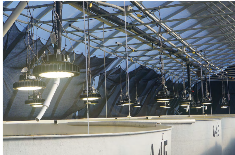
Upgraded 250-watt LED grow lights provide warmth for commercial oyster harvesting tanks while reducing electricity consumption.
