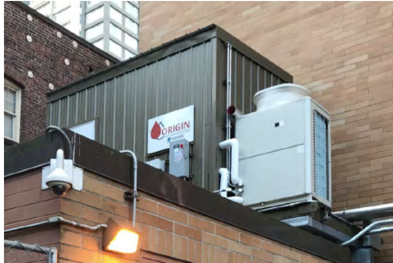
Bayview Towers commercial heat pump water heating system.
