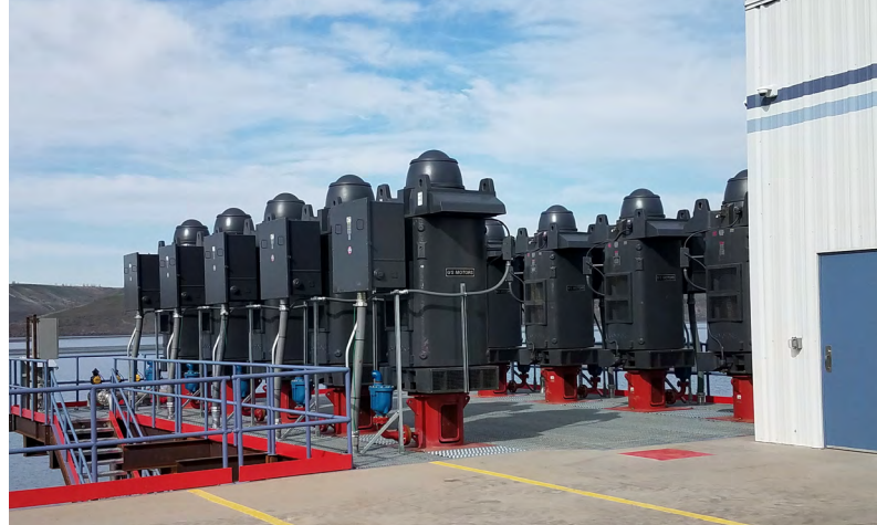
Columbia River pump installation helps recover and stabilize Eastern Oregon aquifers.
