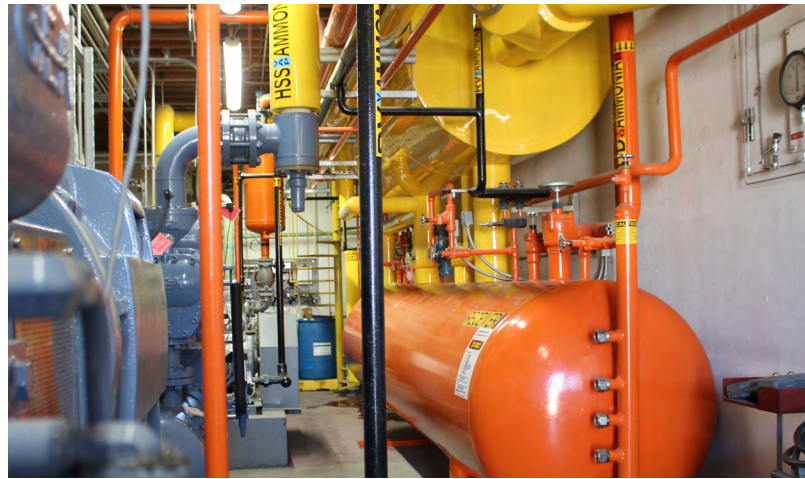
Efficient refrigeration and scrubbing upgrades at a Northern Washington industrial fruit packing warehouse.
