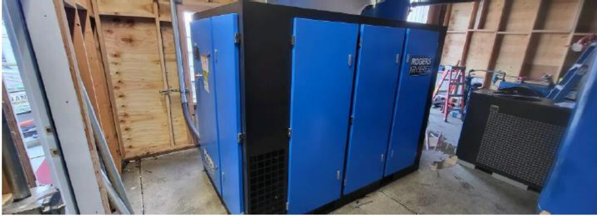
Figure 8-1: New 100 hp VFD compressor
