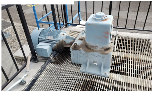
VFD Upgrade on Mixer (operational during summer months only)
