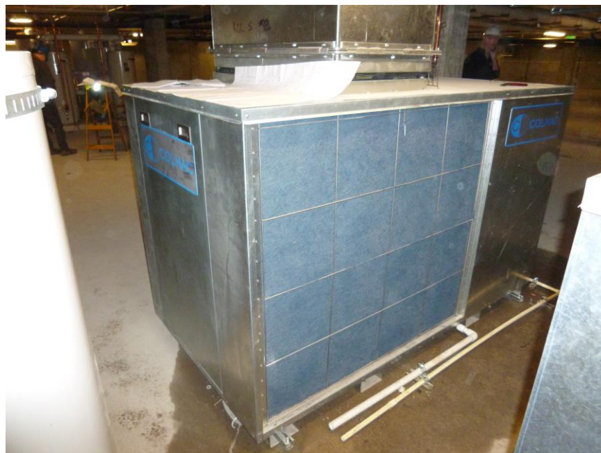
Photo 7: RCC Intake Air Filter
