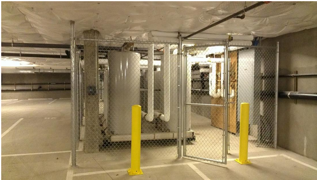
Photo 5: Hot Water Storage Tank Skid
