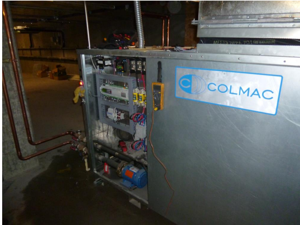
Photo 6: RCC Controls/Pumping Internals
