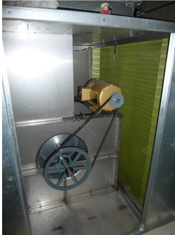
Photo 8: RCC Evaporator Fan and Coil
