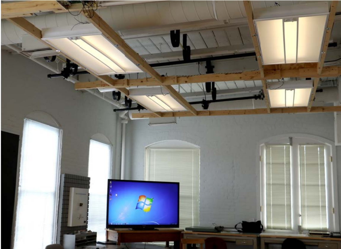
Figure 3: East side of open office with Finelite LED HPR luminaires
