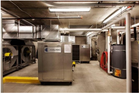
Figure 3: Colmac Industries RCC Equipment
