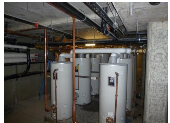
Figure 7: Domestic Hot Water Storage Tanks in Parking Garage
