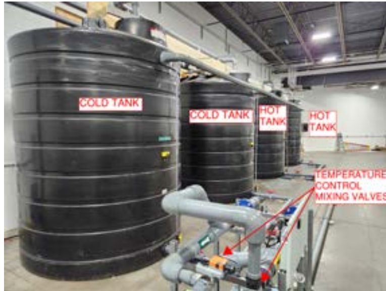
Figure 9. Storage Tanks and Mixing Valves
