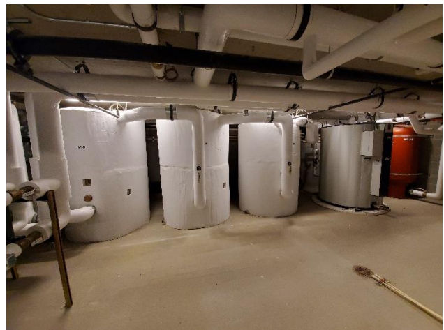
Figure 5. Left to right - primary storage tanks ST8-10 and WH-3 (trim tank)
