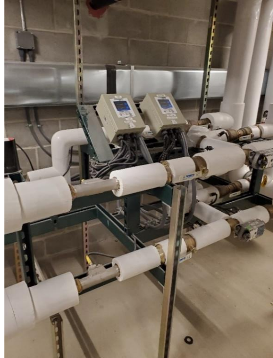
Figure 8. BAS-enabled digital mixing station, yellow thermistor visible in left front pipe
