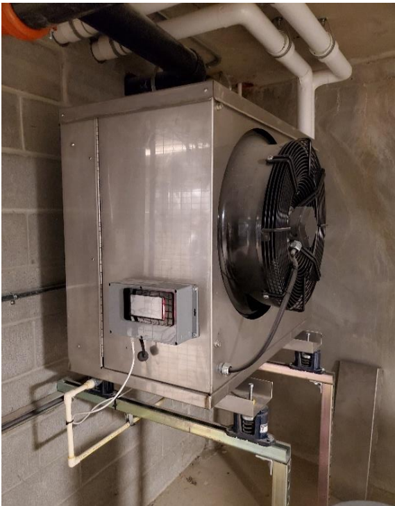
Figure 7. Wall-mounted temperature maintenance HPWH-7 (CxV)
