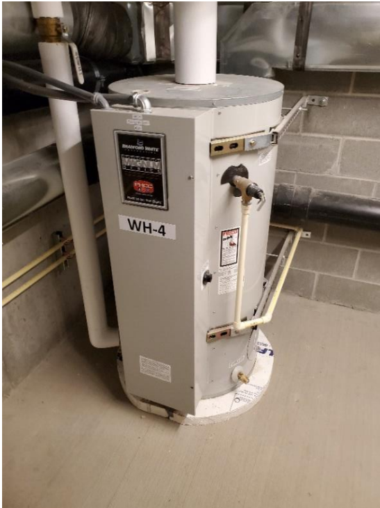
Figure 6. Backup primary electric resistance tank, WH-4
