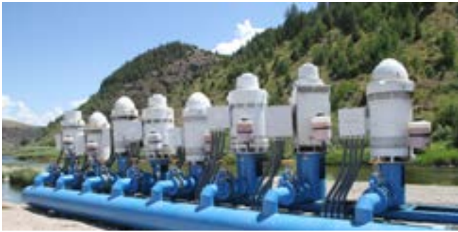
Eight new pumps installed at Schwendiman Farms.
