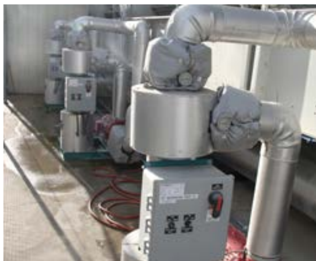
Cooling tower separator pumps installed at the Rainbow Hotel and Casino.
