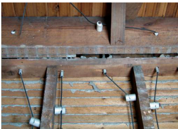
Knob and tube wiring: Obsolete and worn wiring should be replaced during energy retrofit work so that building cavities can be sufficiently insulated.
