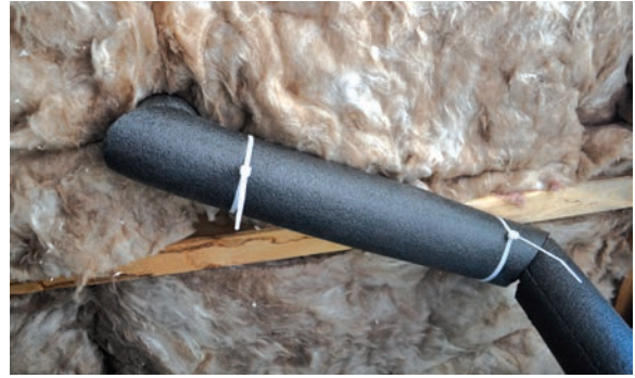
Pipe insulation: Draw bands clamp foam pipe insulation to a hot water pipe.
