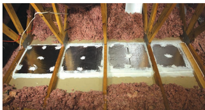
Kitchen soffits: The ventilated attic is connected to the soffit and the wall cavity through framing flaws. Any hole in the soffit creates a direct connection between the kitchen and attic. The photo shows a soffit sealed from the attic with foam board and 2-part spray foam. Image courtesy of Anthony Cox
