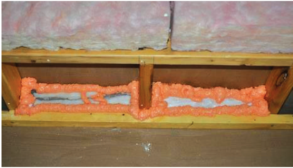
Foam-insulated rim joists: 4 inches of EPS foam is sealed around its perimeter with one-part foam.
