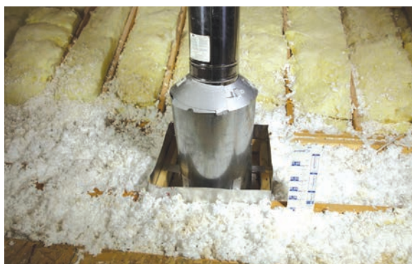
Attic insulation shield: Non-combustible material maintains 3-inch clearance around heat producing fixture and extends above insulation. Image courtesy of Advanced Energy
