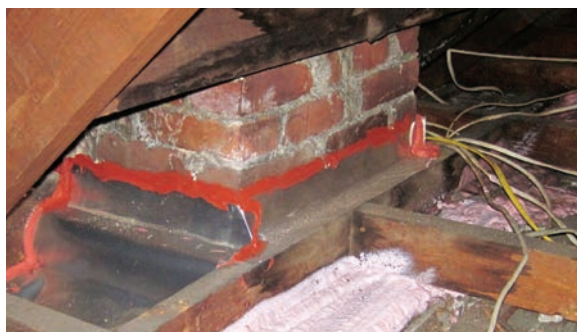
Air-sealed chimney with metal shield: Metal flashing bridges the gap between the chimney and the framing and a metal shield keeps the insulation 3 inches away from the chimney. Image courtesy of Advanced Energy
