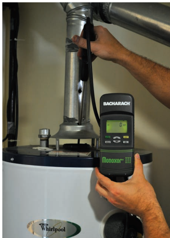
Measuring CO: Measure CO in undiluted combustion gases as they leave the heat exchanger.
