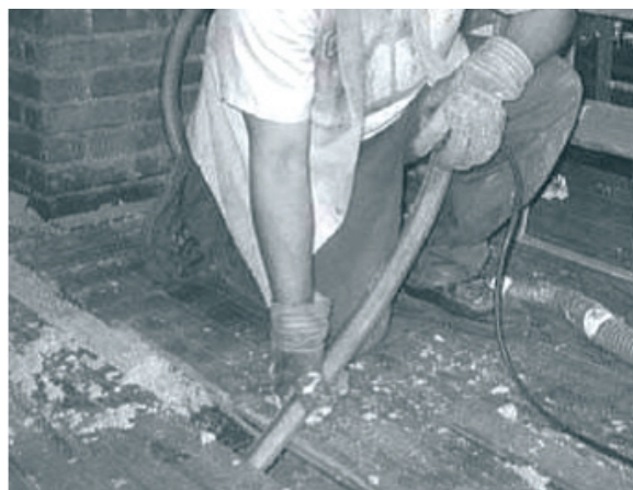
Finished attic floor: Find the large air leaks underneath the flooring and seal them before insulating the space between the joists.
