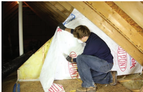
Walls in attic area: Cover new attic wall insulation with a durable, vapor-permeable air barrier to prevent air penetration of the insulation and to ensure that the insulation is held in full contact with the wall. Image courtesy of Energy Smart Academy
