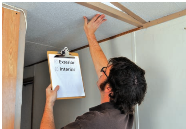
Preparing to blow a manufactured-home roof: Inspect the ceiling to be sure it can support the weight of more insulation. Image courtesy of Energy Smart Academy
