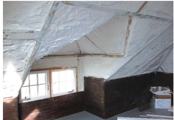
Unvented attic: Insulate the roof decking with an air-impermeable vapor barrier. Image courtesy of Neil Kelly
