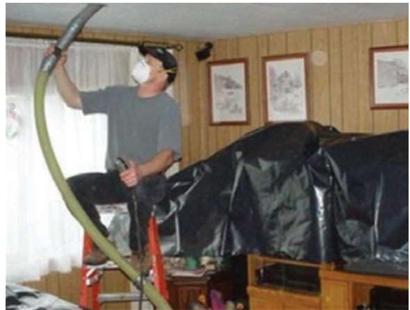
Blowing through the ceiling: The contractor pushes the fill-tube into the cavity and out near the edge of the roof. The holes are drilled in a straight line for appearance.
