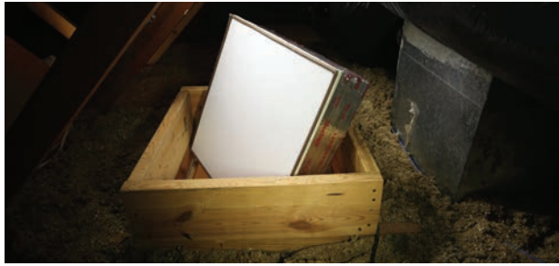
Insulated attic hatch: Building a dam prevents loose-fill insulation from falling down the hatchway. Foam insulation prevents heat transfer through the access hatch. Install insulation to achieve attic insulation R-value of R-30. Image courtesy of Energy Smart Academy
