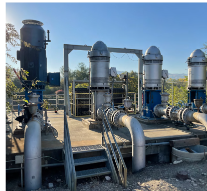
New 800hp stainless steel pumps (blue)
