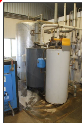
Hot Water System
