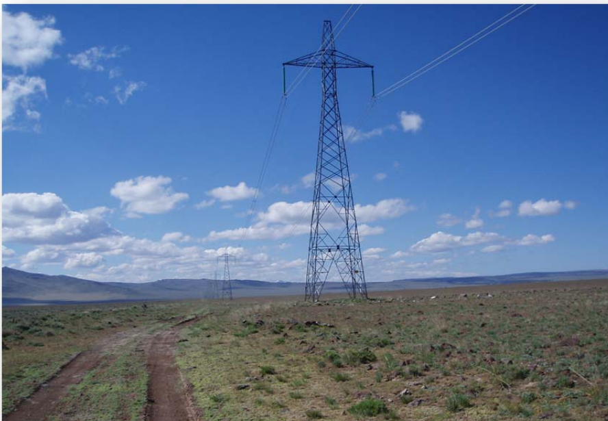
Figure 2.1-5: Existing PDCI Line BLM Land South of US 395 (Tower 220/2 looking south)
