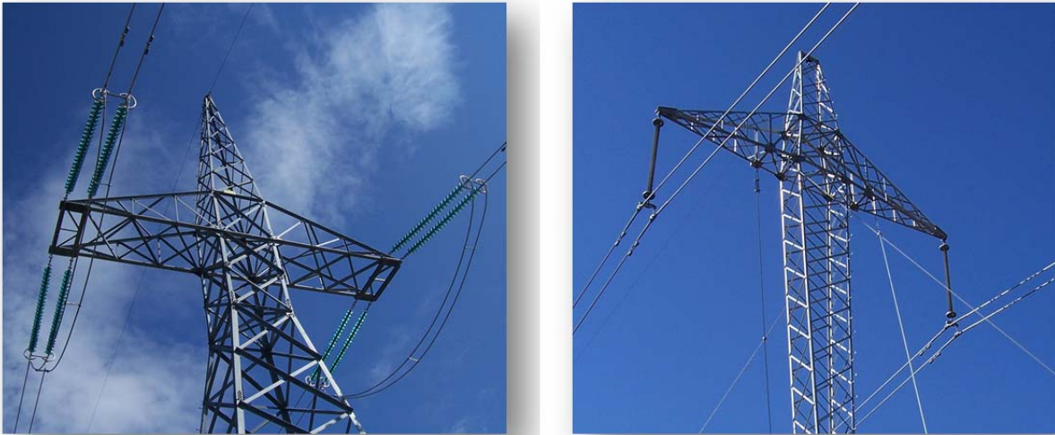
Figure 2.1-7: Glass Insulators on Dead-end and Rigid Insulators on Guyed Tower
