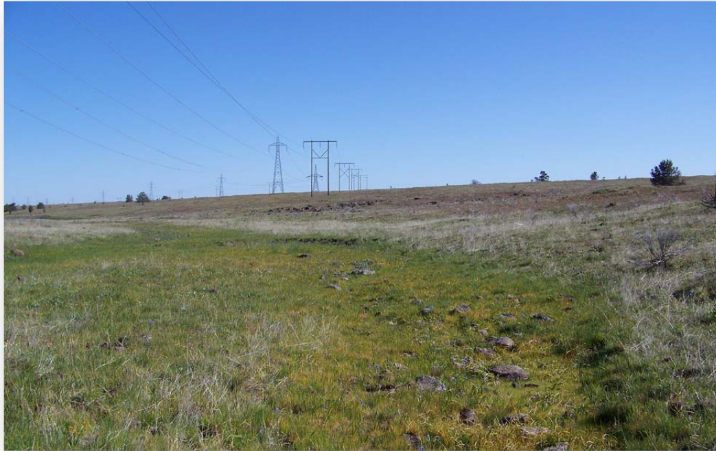
Figure 2.1-2: Existing PDCI Line North of US 97-US 197 Intersection (looking north from Tower 48/1, Big Eddy-Redmond No 1 is on the right)
