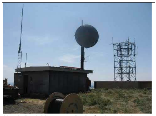
Mary's Peak Microwave Radio Station, viewing sou
