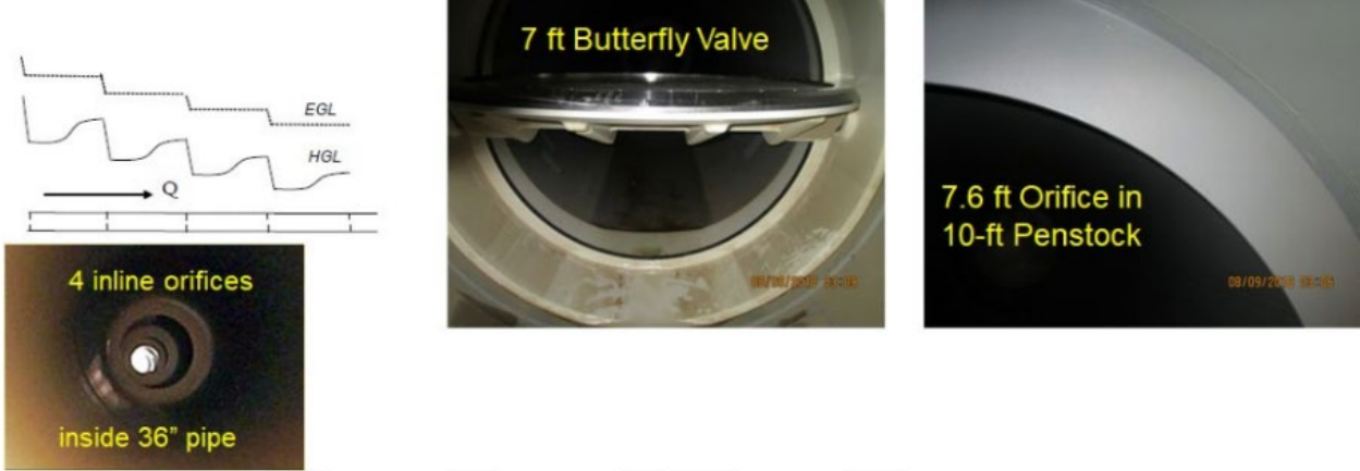
Figure 1-3 In-line Orifice Systems inside Pipelines (Seven Oaks Dam, lower left; The Dalles Dam, upper middle and right)
