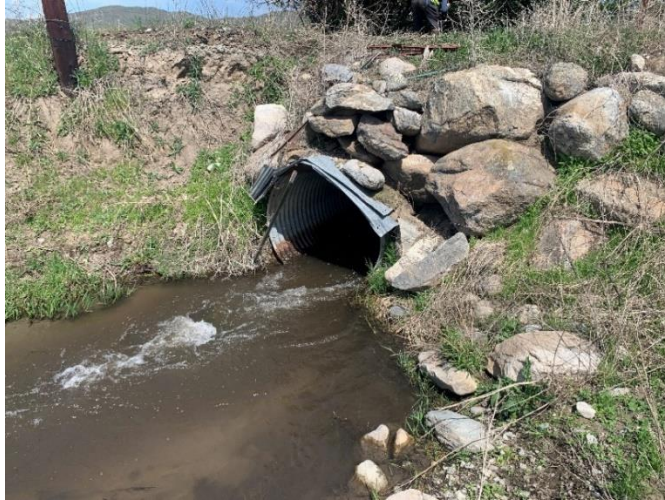
Figure 5. Photo of the outlet of the existing pipe culvert to be abandoned at the downstream end of the Barn Field reach.
