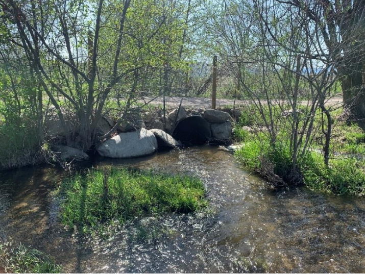
Figure 3. Photo of the inlet to the existing pipe culvert at Whiskey Creek Road in the Upstream sub-reach.
